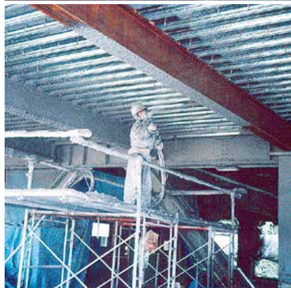
Top: Reputable hardware (continuous mixer) is deployed; Bottom: A proper and safe job site setup is crucial in achieving the product's designed in-place performance and in meeting the construction schedule.
